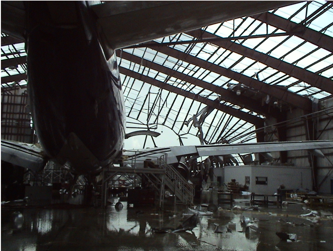
Damaged aircraft in destroyed hangar at Baton Rouge, LA following Hurricane Rita. Photo by CPT Marcel Minutolo, taken while on duty performing relief operations following Hurricane Katrina in 2005.
